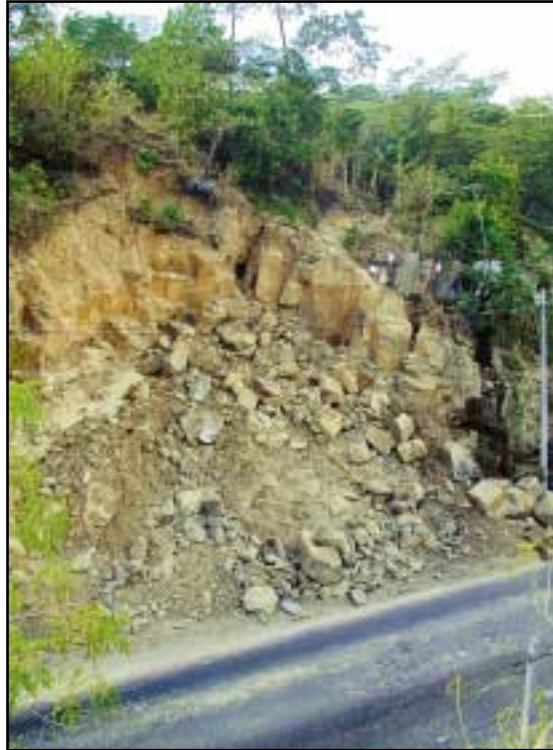
Figure 7. Rock fall between Zaragoza and El Transito.
