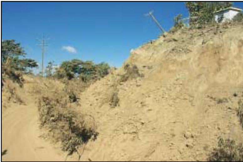
Figure 11. Road-cut failures on road from Las Delicias to Comasagua.
