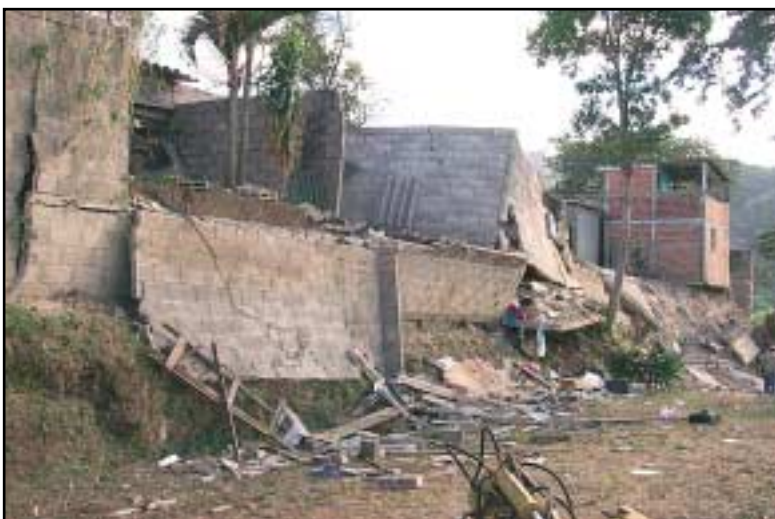
Figure 12. Damage from strong shaking and landsliding at Alpes Suizos.
