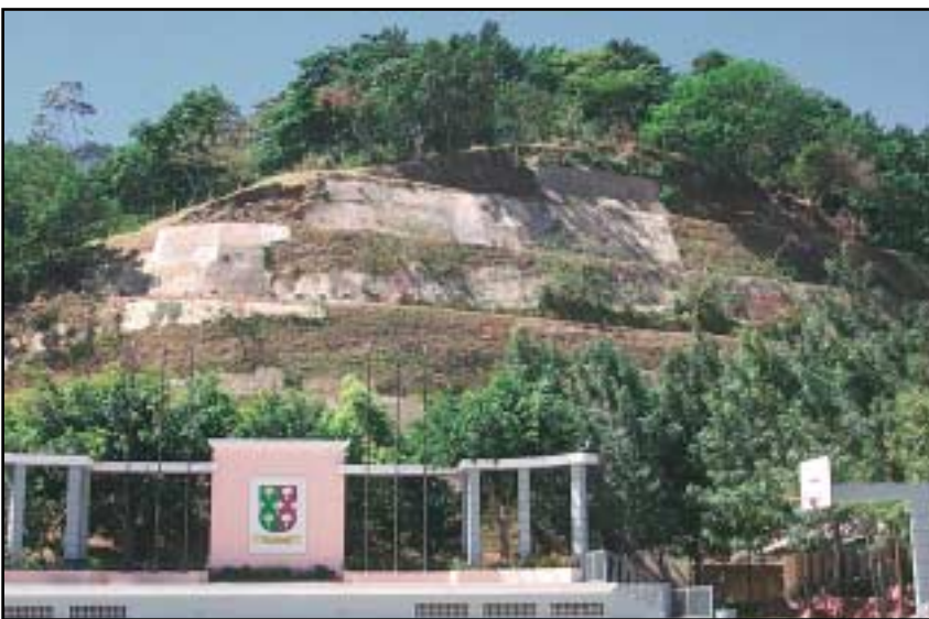
Figure 6. Cut slope above La Floresta school for girls. Scar on upper left part of slope is a small landslide triggered by the January 13 earthquake.
