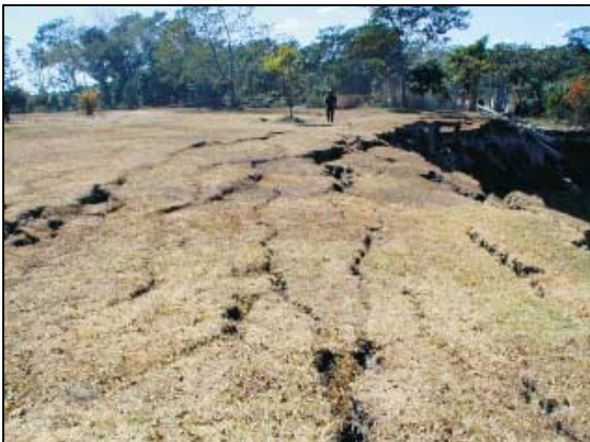
Figure 3. Cracks above head scarp of Las Colinas landslide.
