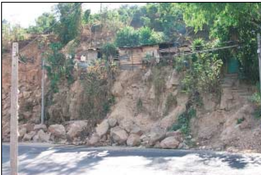
Figure 8. Houses along rock-fall scarp between Zaragoza and El Transito.
