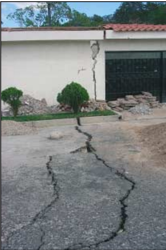
Figure 13. Cracks along the edge of a fill slope at La Cima 3.
